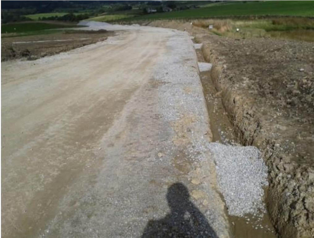
Plate 3.6: Check dam example
