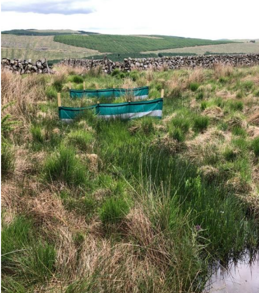
Plate 3.4: Typical silt fencing
